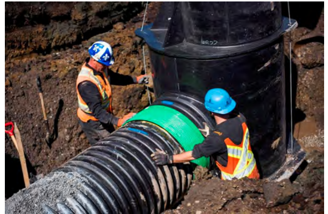
Connection of the large diameter HDPE pipe to manholes was easy and efficient at the site.
