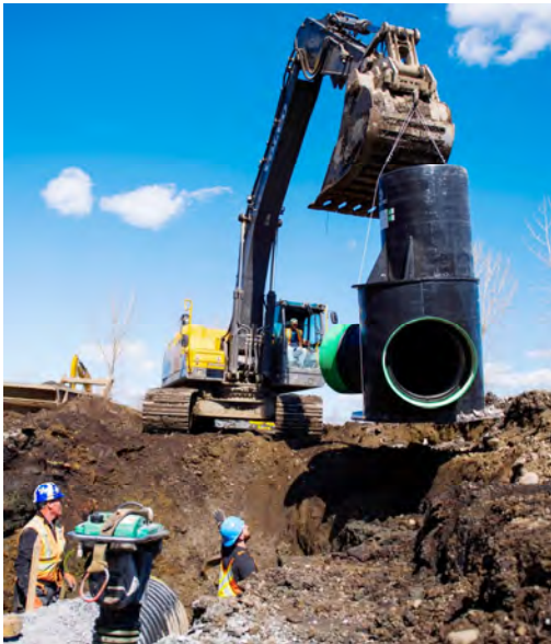
Inlets and outlets were added to the HDPE manholes at the factory, which sped installation.
